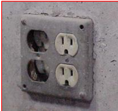
Loose / Recessed Receptacle
